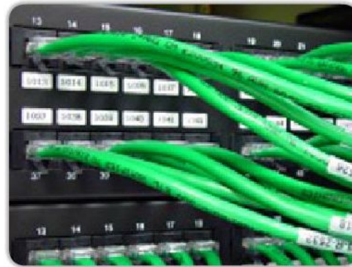
Front of Patch Panel
