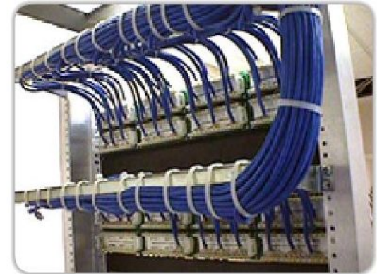
Rear of Patch Panel
